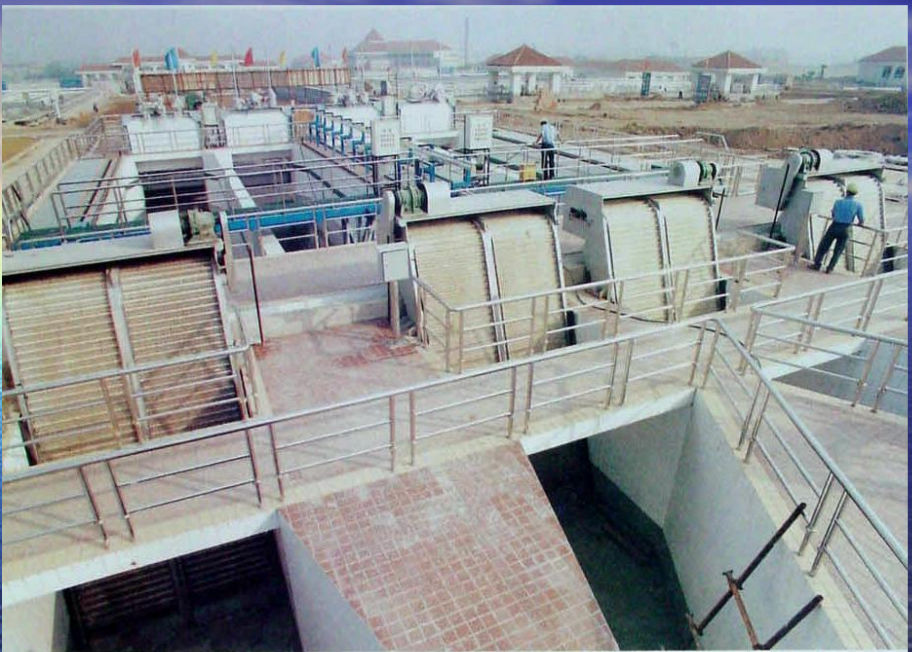
Grilles and Grit Setting Chamber of Nanjiao Water Treatment Plant
